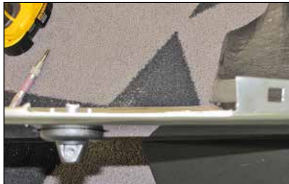
53. Using a cut-off wheel or similar tool, cut along the lines marked with the template and remove that section of the fender. Be sure to remove any remaining burrs with a file or deburring tool.
